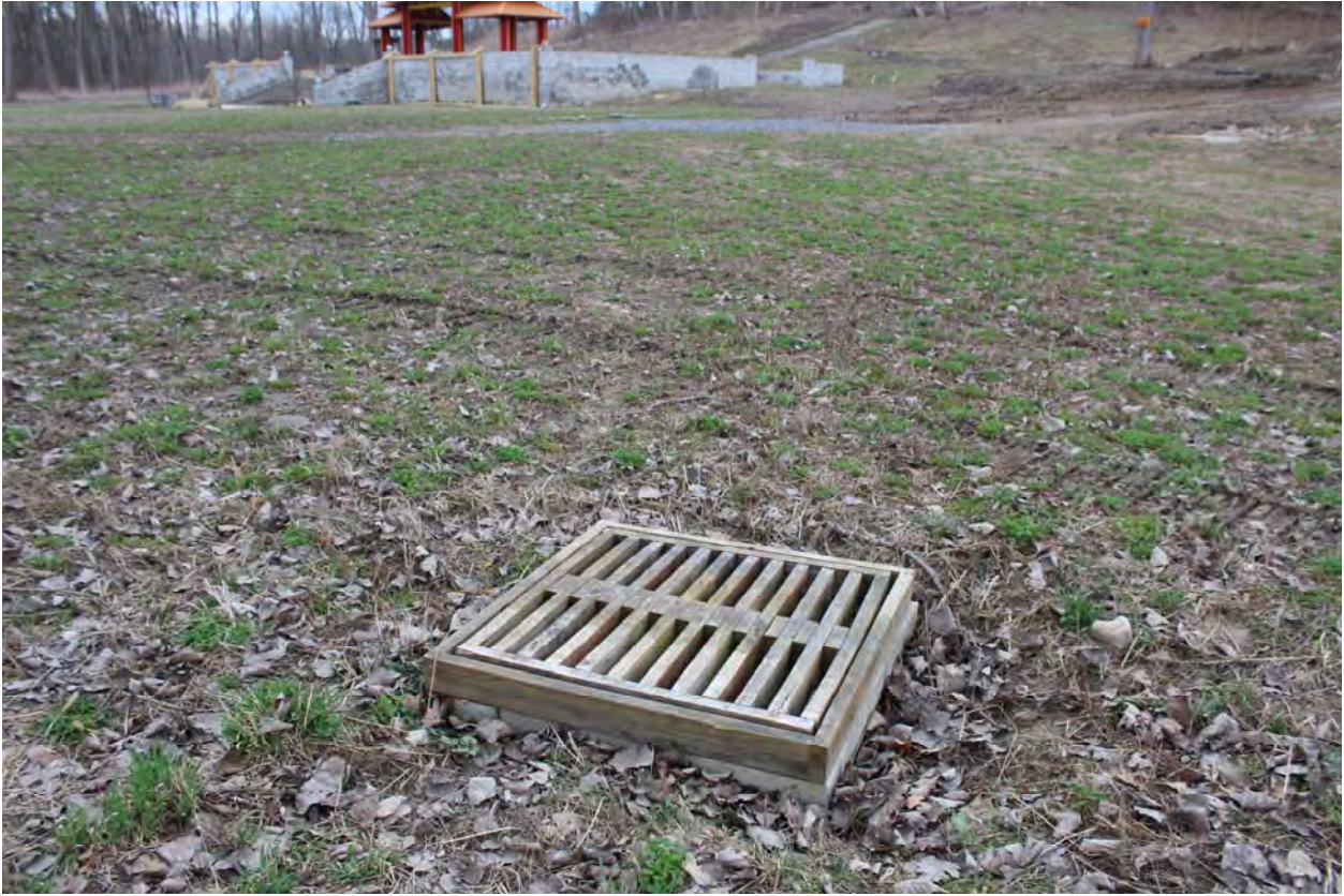
Photo 11. View of stormwater drain in the central part of Area 1, facing east.
