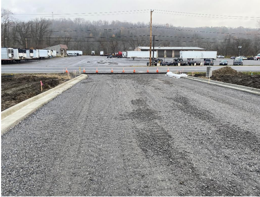
Figure 1 - View of subbase grading and new curb for western driveway, looking northeast.
