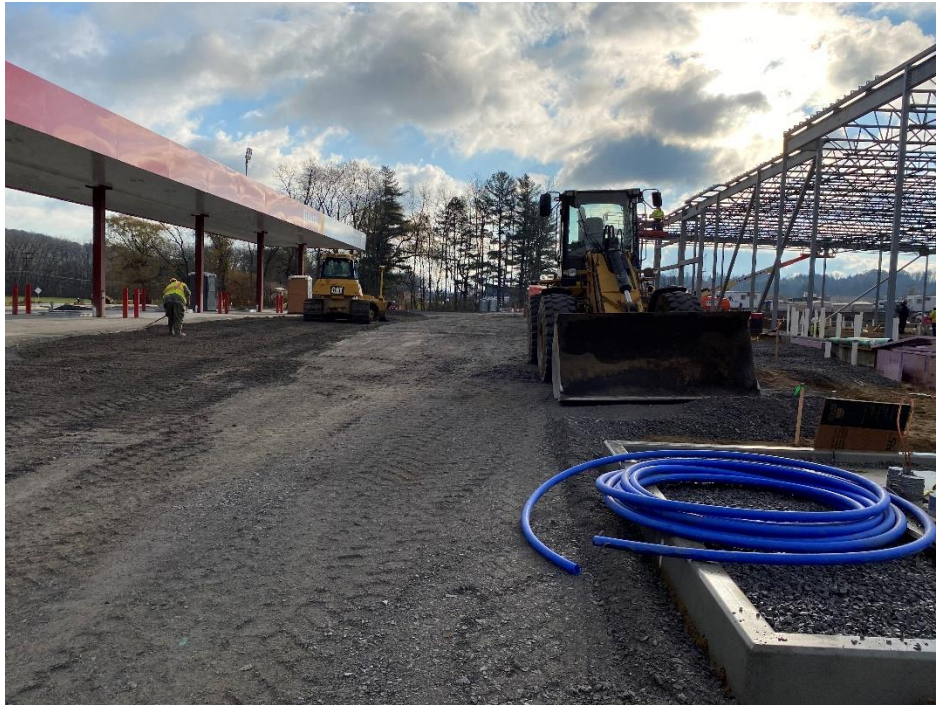
Figure 3 – View of subbase grading for front parking and fuel pumps, looking east.
