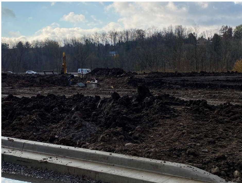
Figure 4 – View of grading and outlet structure for southern stormwater pond, looking southeast.
