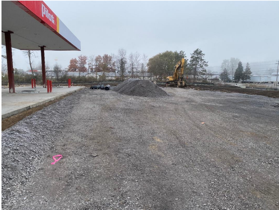
Figure 3 – View of subbase grading for front parking and fuel pumps, looking west.
