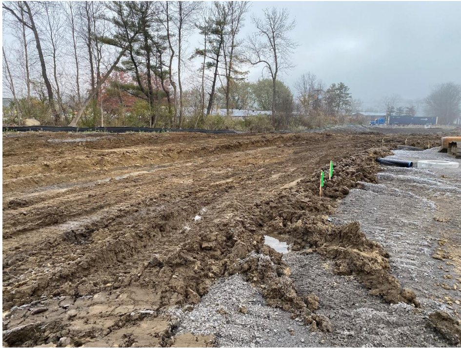
Figure 5 – View of grading for bioretention area along west side of site, looking northwest.
