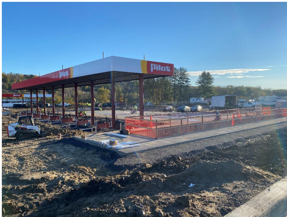
Figure 4 - View of truck fuel pump area, looking northeast.
