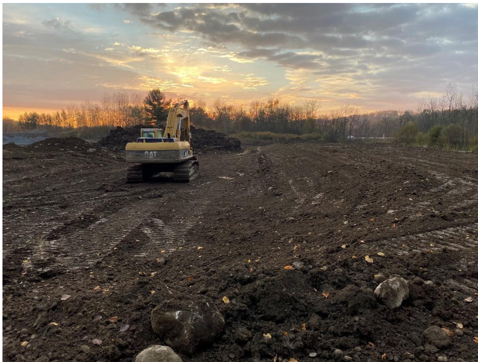
Figure 4 - View of grading for stormwater pond at south end of site, looking east.
