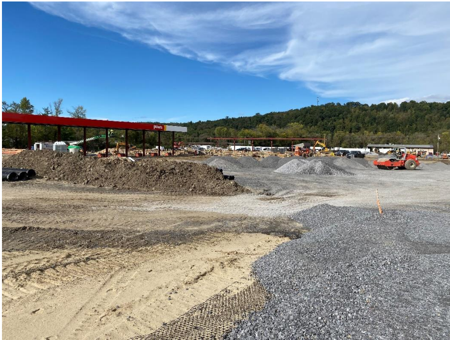
Figure 1 - View of grading and steel erection for truck fuel pump area, looking north.
