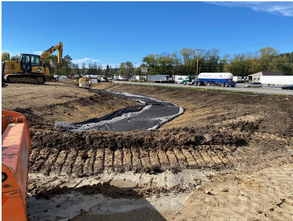
Figure 4 – View of grading for east bioretention pond at north end of site, looking northwest.
