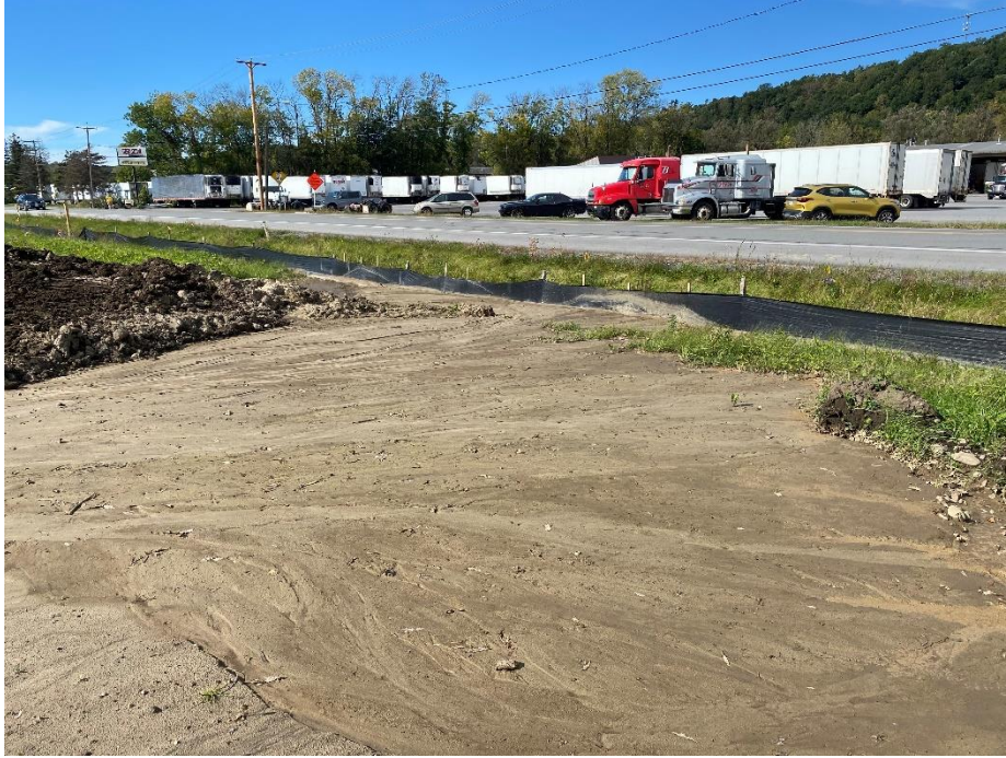
Figure 1 - Clean out silt from along silt fence at north end of site.
