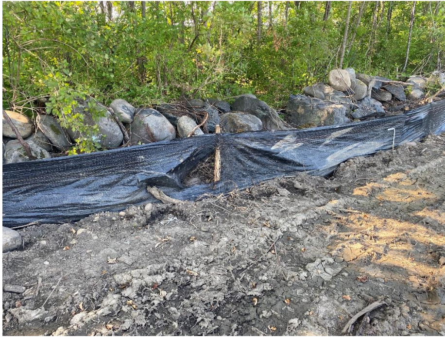
Figure 1 -Hole in silt fence along western side of site, need to replace section.
