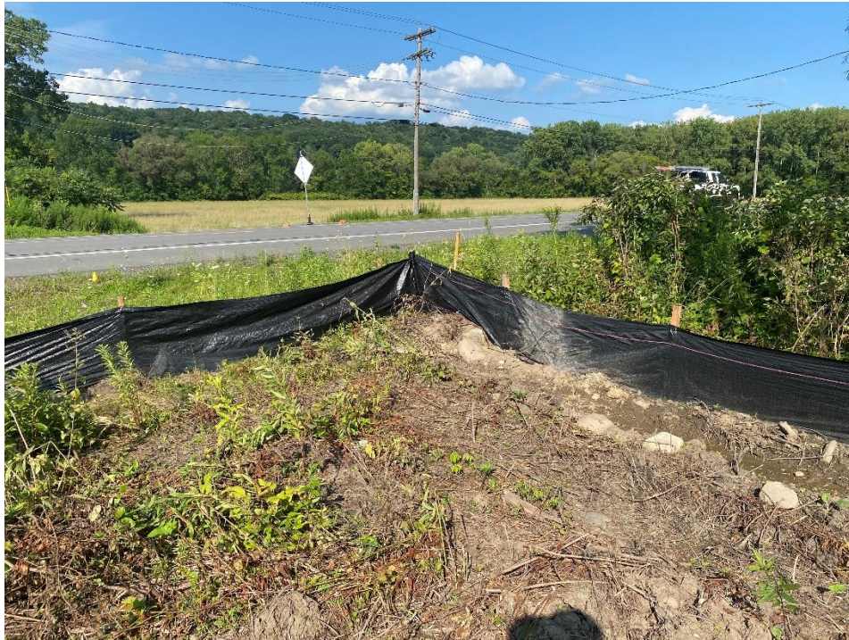
Figure 5 – Repaired silt fence in NE corner of site.
